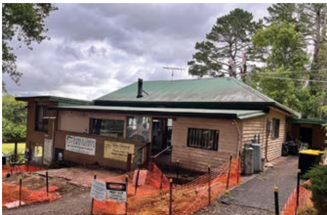
Photo: The renovated club house will be accessible by a ramp once completed.
